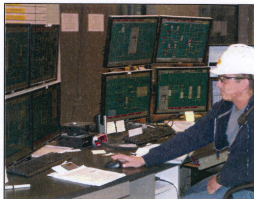
Matt Adams, lead operator, checks operations in the control room.
